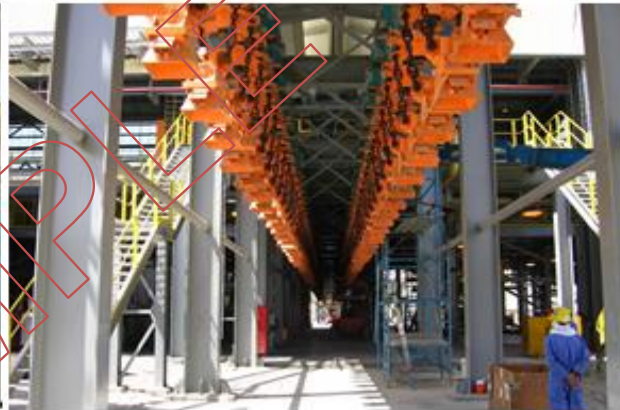
Power & Free conveyor system
